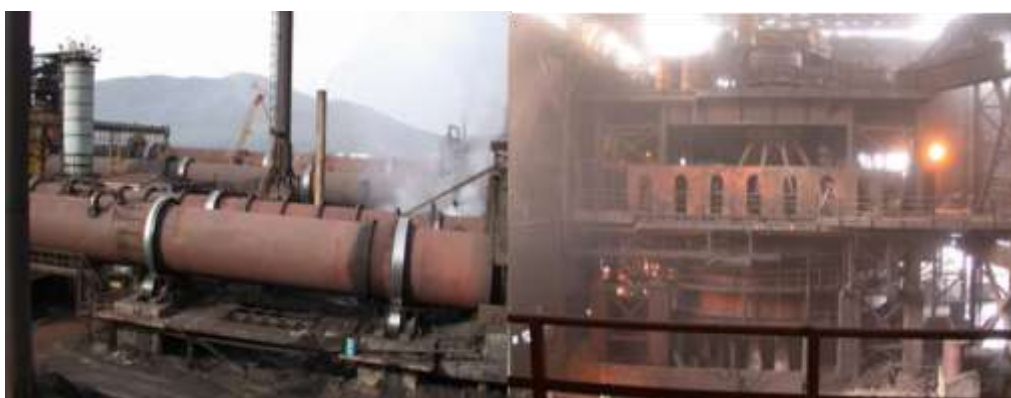
Figure 28. Rotary Kiln (R/K) (left) and Electric Furnace (E/F) (right) at the metallurgical plant.
