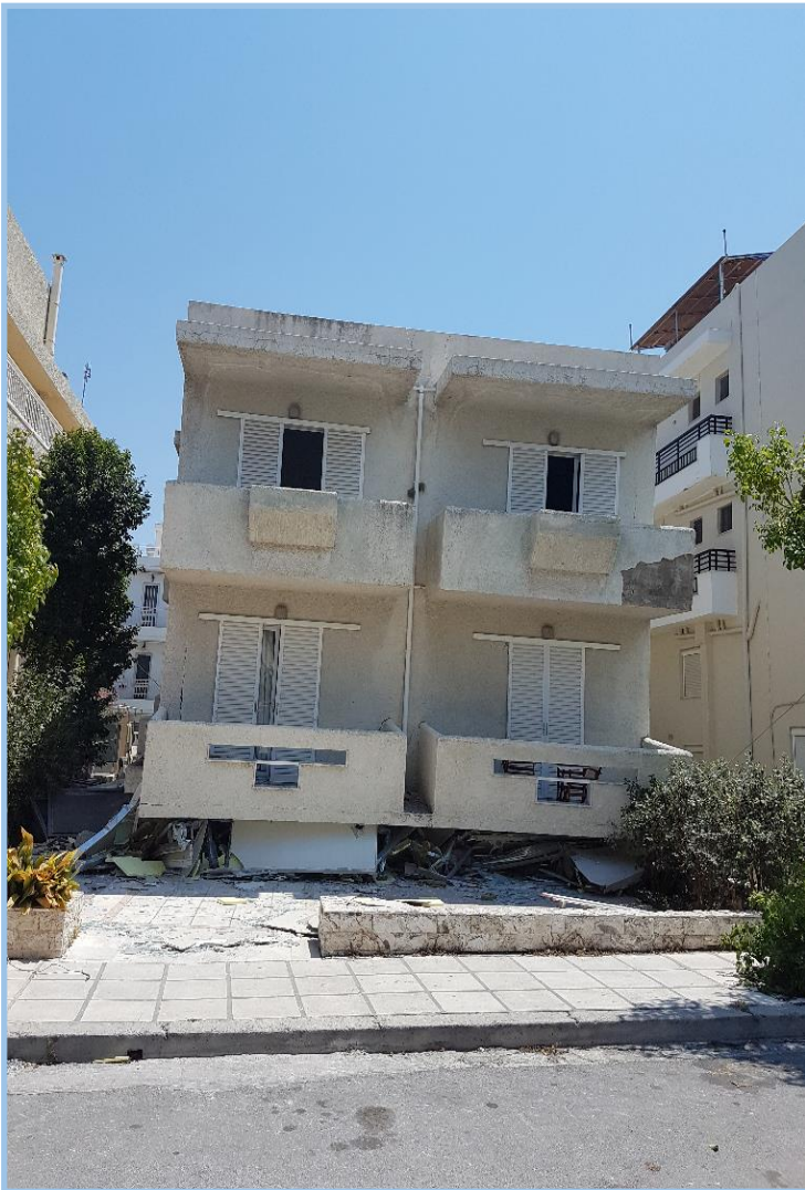
Two stories were added at a later stage on an existing weak ground floor. The ground floor totally collapsed being squeezed, while the two upper stories suffered relatively no damage.
