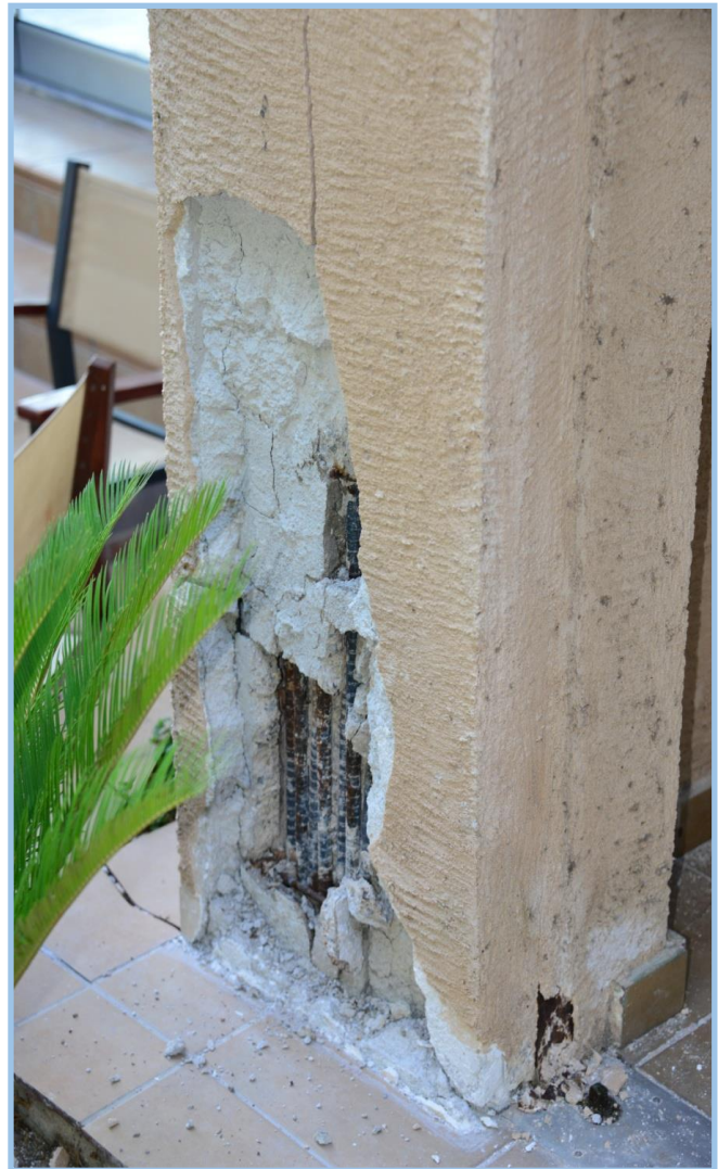
Spalling of the concrete cover attributed to concentration of many steel bars without retaining the appropriate distance among them. Steel corrosion and the resulting bloating of bars is also observed.
