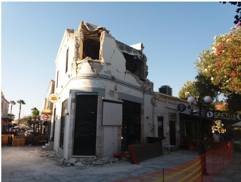
Figure 5.10. A masonry building that survived the 1933 earthquake in the historical center of Kos city. The partial collapse of the upper floor with the 2017 earthquake killed two persons.
