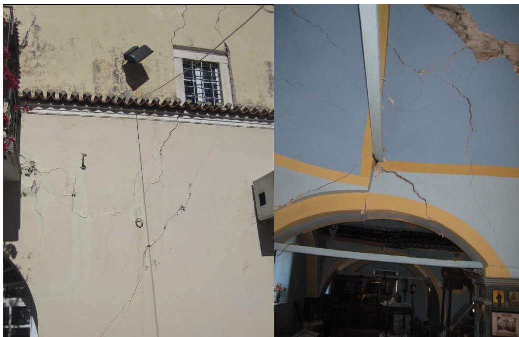
Figure 5.6. External and internal damage at the Church of Christ in Ano Vathy, Samos, after the earthquake ( M_w=7.0 ) of 30 October 2020 (photos credit, I. Triantafyllou).
