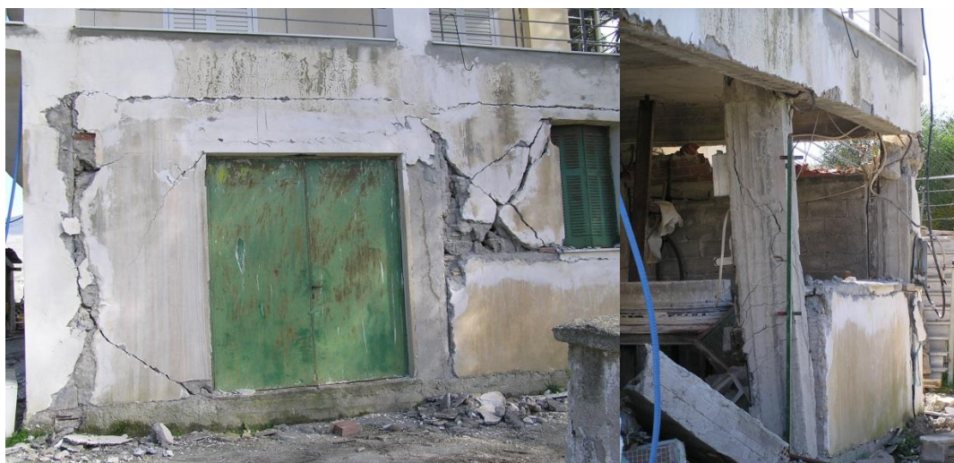
Figure 5.2 Damage in a two storey building in Ayios Dimitrios, Cephalonia Island, after the 26 January 2014 ( M_w=6.0 ) earthquake (left) and after the 3 February 2014 ( M_w=5.9 ) earthquake (right) (photos credit, I. Triantafyllou).
